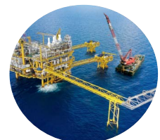
Off-shore fire protection system
